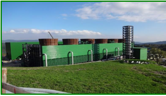
Figure 6: Bagnore 4 (40MWe) power plant.
