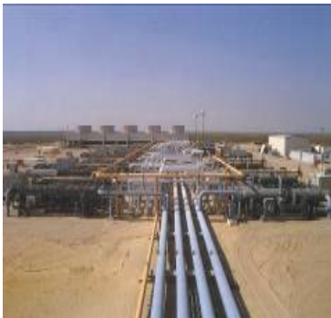
Fig. 8: ORMESA I, Cal., USA, 30 MWe
